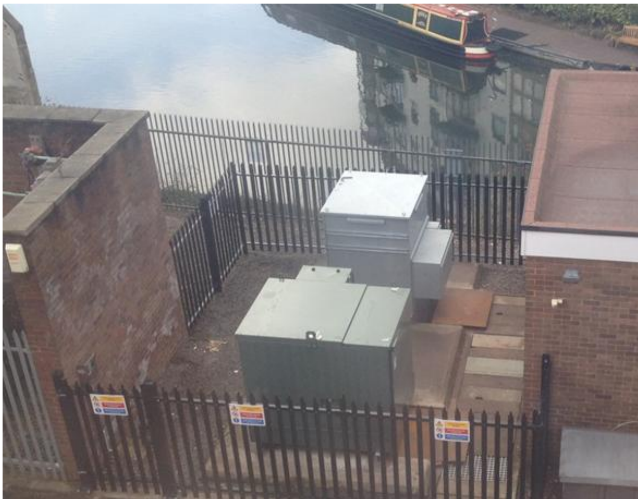
Ladywood FLM Installation
