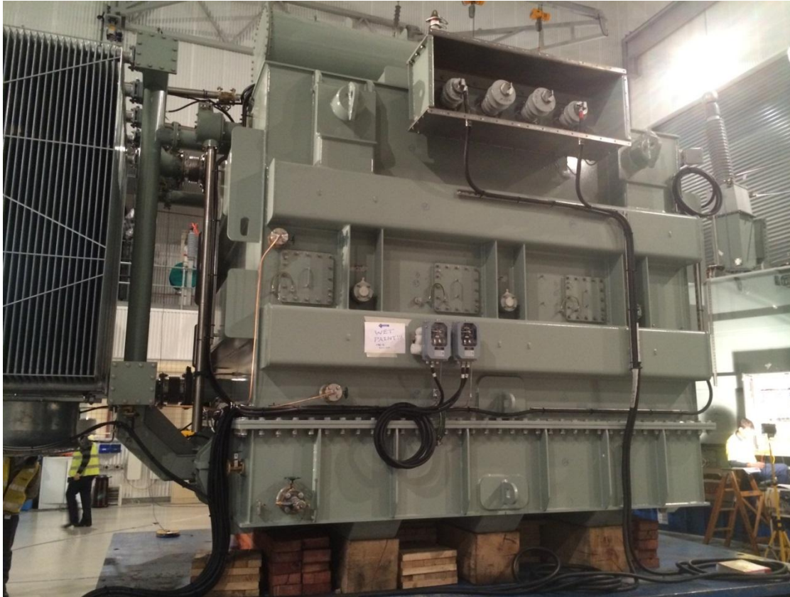
GridON FCL – During Factory Acceptance Testing
